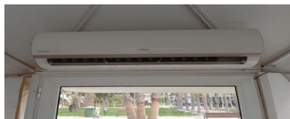
Figure 4 Air conditioner deployed in Smart Home
